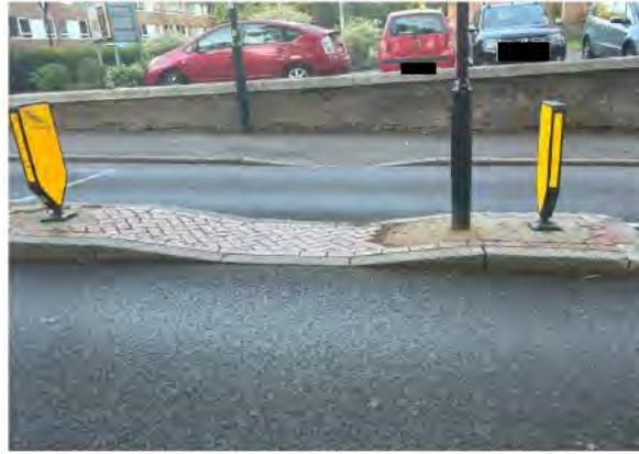
Photo 1: Existing dropped kerb
